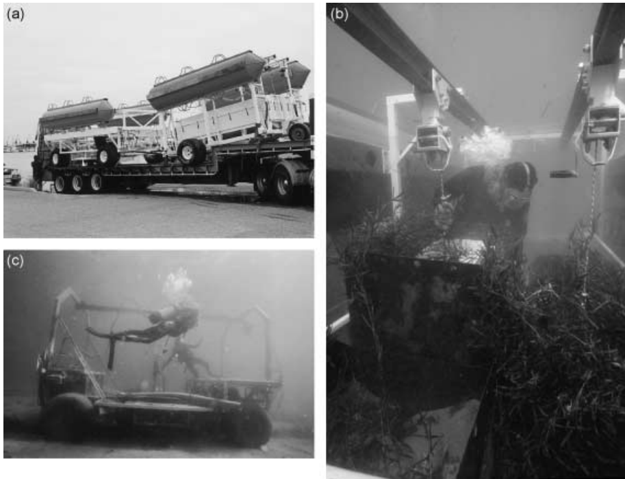
Figure 3. The need to salvage large areas of seagrass as a result of sand mining operations in Western Australia led to the development of submersible machines (such as ECOSUB1 and 2) capable of transplanting large sods of seagrass. The main advantage of large sods is that they have a greater mass and a better rate of survival in high wave energy environments compared with those transplanted by hand. Clockwise from top left: (a) ECOSUB2 and accompanying sod shuttle prior to launching (photo reproduced with permission of Cockburn Cement Limited, Western Australia); (b) a diver storing a seagrass sod in the ECOSUB2 sod shuttle at Success Bank in Western Australia; and (c) commercial divers operating ECOSUB2 underwater (photos courtesy of Brian Richards, Murdoch University).
